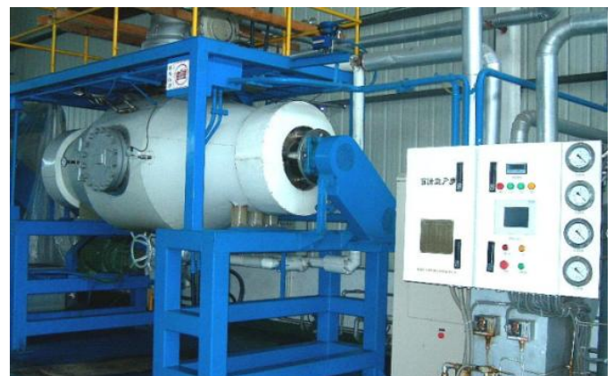
Fig. 2 Subcritical water treatment reactor
