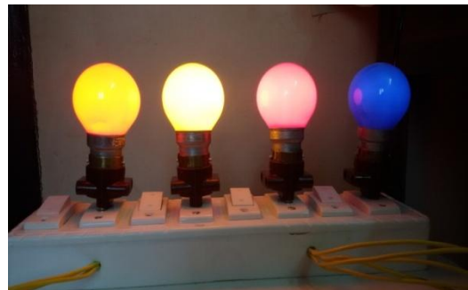
Figure 13:- Two-way switch board is used to switch ON/OFF devices
